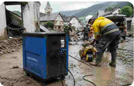
Construction Power Support
